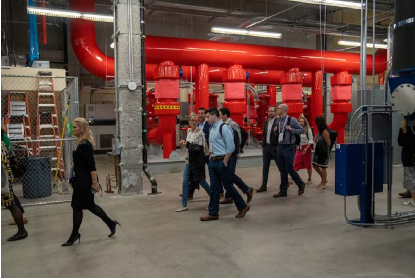
Annual Meeting Visit to Resorts World Las Vegas Facility - Cogeneration Gas Plant Generating Electricity, Heating, and Cooling at Same Time (October 23-26, 2022)
