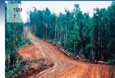
Regeneration of the crude oil export pipeline ROW approaching Mubi valve station. May 1998
