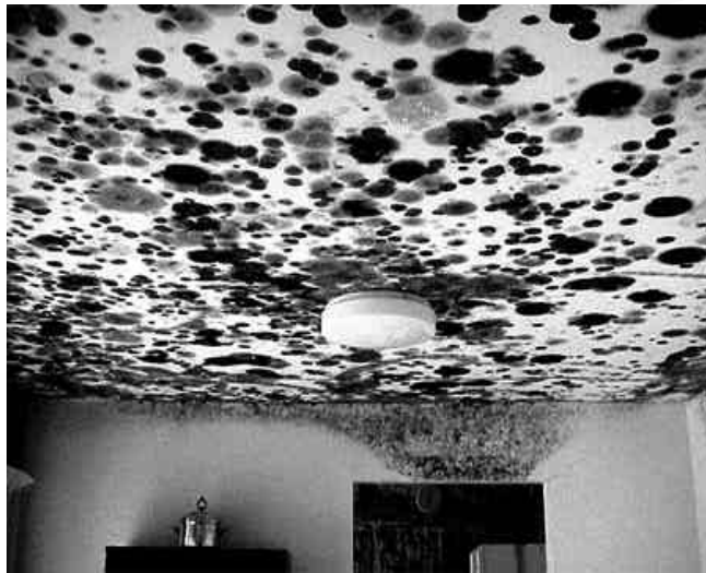
Mold on Ceiling
